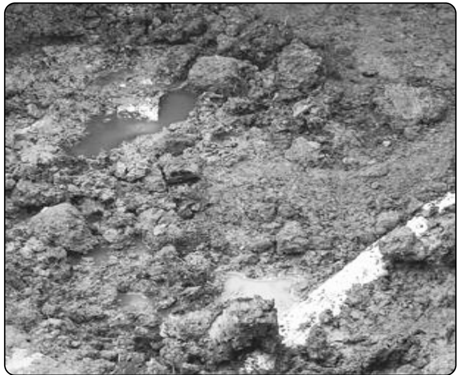
Wastewater rising to the surface or "ponding" as a result of a failed drainfield.
