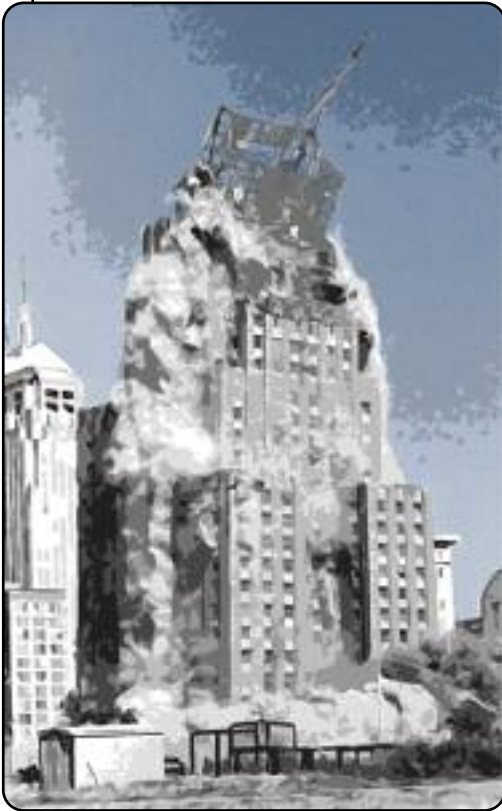
Controlled demolition of abandoned buildings creates tons of rubble. If graded and sized properly, this waste material can be used as a substitute for native gravel in drainfields.
